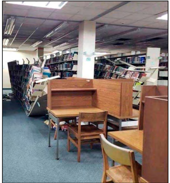
Earthquake damage from Pontifical Catholic University of Puerto Rico, Encarnacion Valdes Library.
