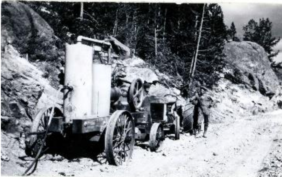
Early road construction technology. Air compressors that powered pneumatic drills on Fall River Road
